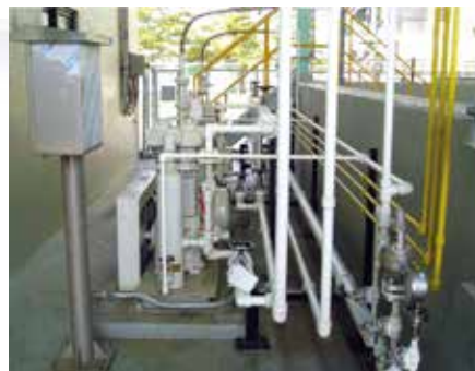
Ammonia unloading compressor
