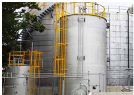
Aqueous ammonia storage tank
