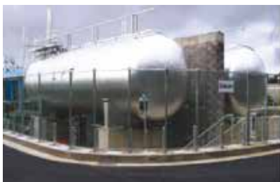
LPG storage facilities
