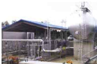
Mixed gas supply equipment
