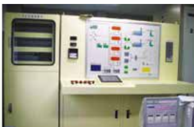
Main control room
