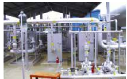
LPG vaporization and mixed equipment
