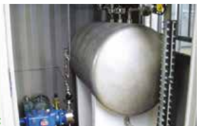
Odorant injection equipment
